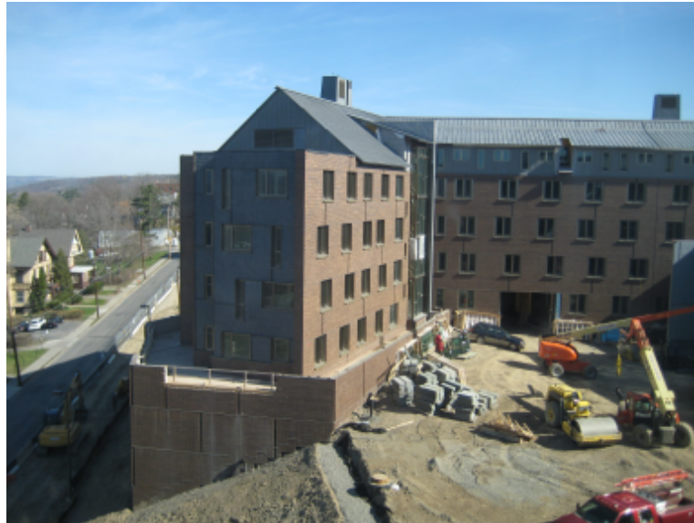
Residential Bar – View showing steel framed gabled roof on top of precast plank and bearing wall building.
